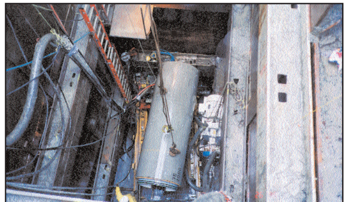
Right: A 10-ft section of 36-in. RCP is placed into the jacking frame during heavy El Nino rains.
