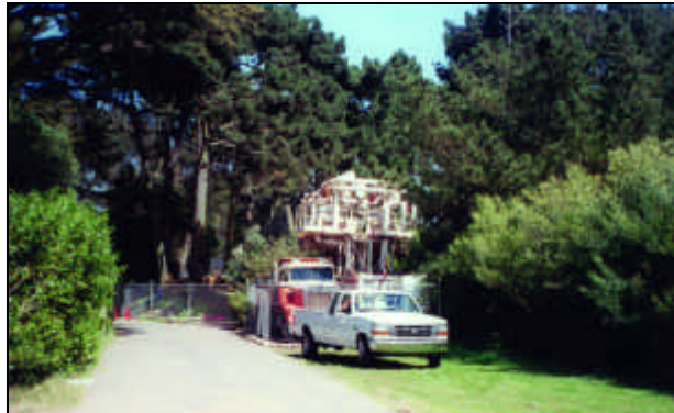
This project in the San Francisco Zoo demonstrated microtunneling’s ability to minimize disturbance.
