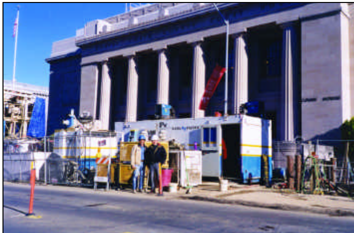
Nada Pacific completed the Martinez East Side Sewer Improvement Project through busy areas of Martinez, Calif., including in front of the Contra Costa County Courthouse.
